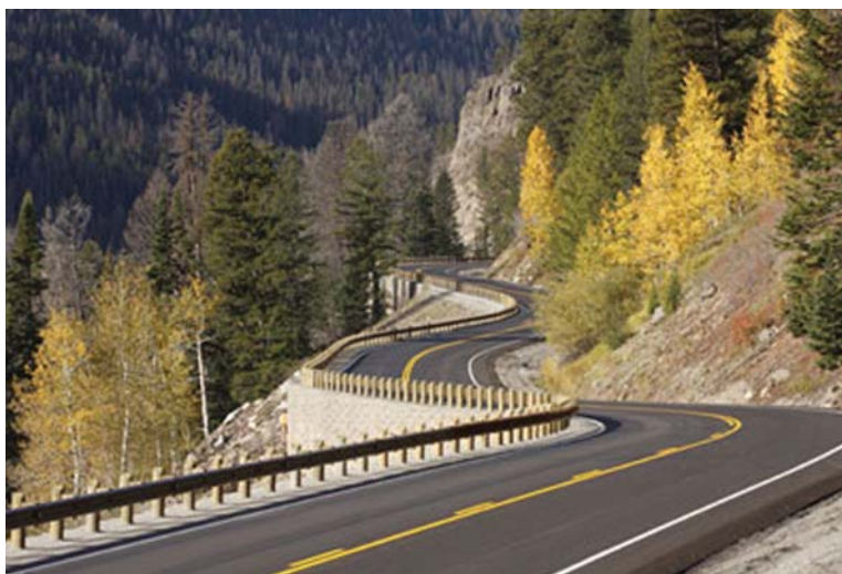
A section of the East Entrance Road to Yellowstone National Park in Wyoming was paved in August 2007 using warm-mix asphalt.
