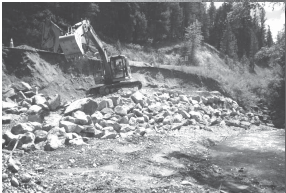
Photos by Tim White, Road Foreman, District #3, Lincoln County Just east of Eureka, Montana Sinclair Creek Road, June 15, 2006, after 7 inches of rain in less than 24 hours
