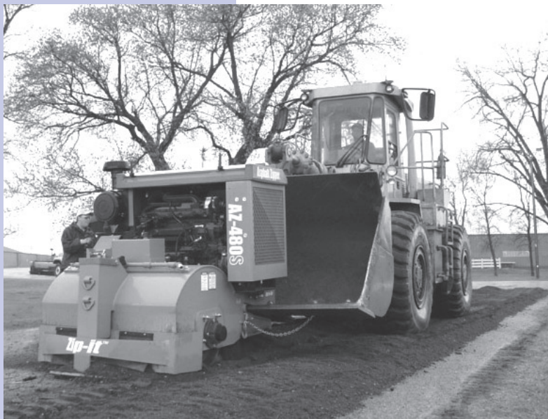
Full depth milling on a deteriorated asphalt street
